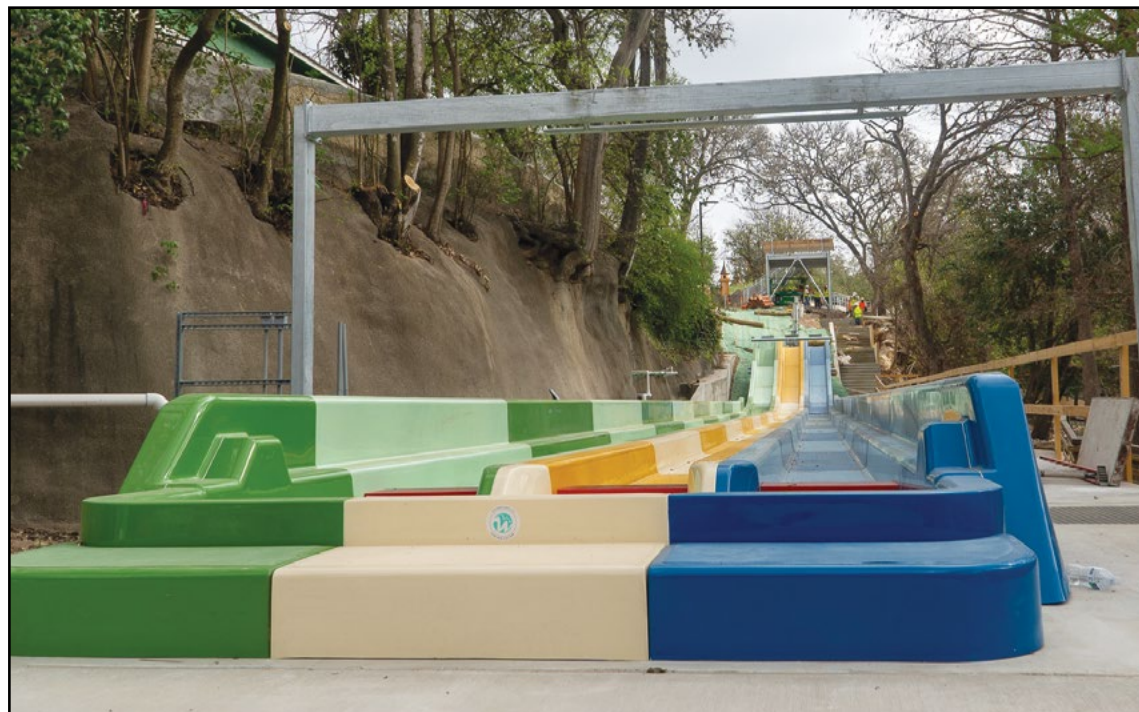
Construction is moving along at a rapid pace. COURTESY SCHLITTERBAHN WATERPARKS & RESORTS
