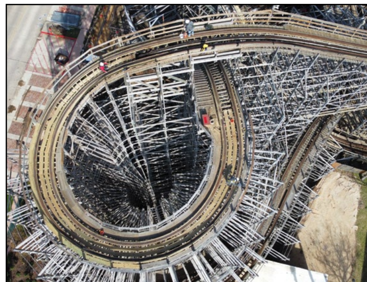
This aerial view shows work being done on the first turn off the lift. .COURTESY TEXAS SKILLED CARPENTRY
