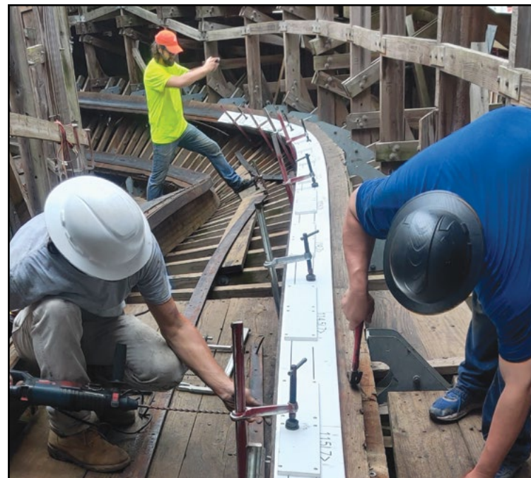
The team from Texas Skilled Carpentry — who has worked with the park for more than a decade — works on trouble spots to keep Boardwalk Bullet in top condition. COURTESY TEXAS SKILLED CARPENTRY
