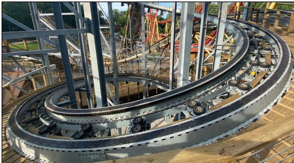
The combination of Titan Track and steel supports in the layout made the spiral lift possible. AT/GARY SLDE
