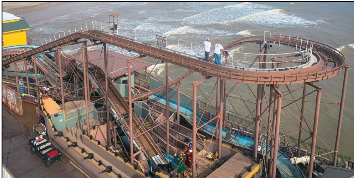
The flume at Galveston Island Historic Pleasure Pier is receiving TLC, after the facility's coaster did in 2022. COURTESY BAYNUM SOLUTIONS
