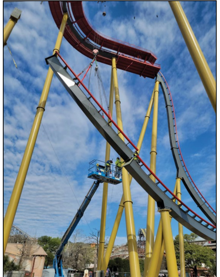
Construction on the B&M coaster took place in the center of the park during operating days. COURTESY NORTHWEST COASTERS
