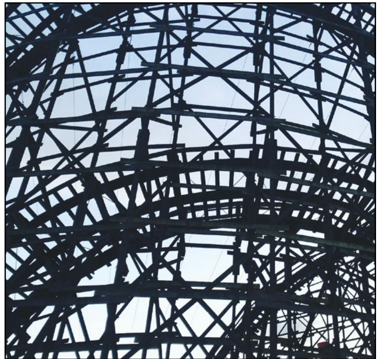
Playland's Wooden Roller Coaster is made entirely from Douglas Fir. And that is what Martin and Vlemickx Rides (MVR), the lead engineering firm for the restoration, used to replace some pieces. COURTESY PNE
