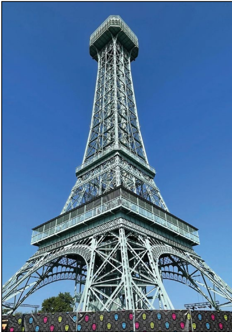
It will take Baynum Painting about 12 weeks to finish the 300-foot-tall Eiffel Tower repaint for Kings Island's 50th anniversary in 2022. COURTESY BAYNUM PAINTING
